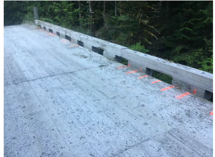
Locations with Pockets of Rot Noted in Ties Adjacent to Riser
