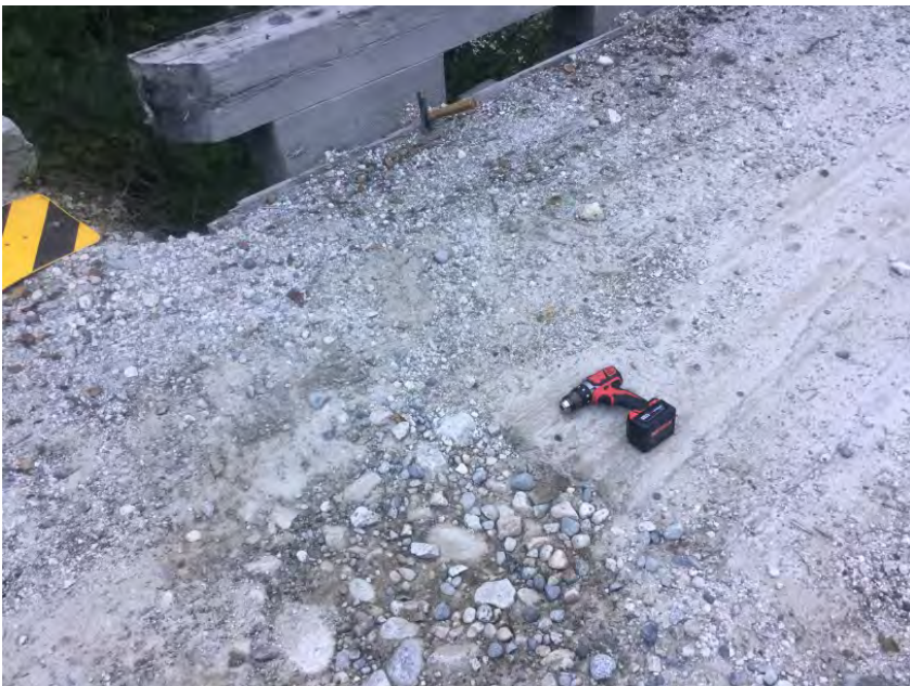
Rotten Deck Plank & Pothole in Approach Producing Heavy Wear in Deck Plank
