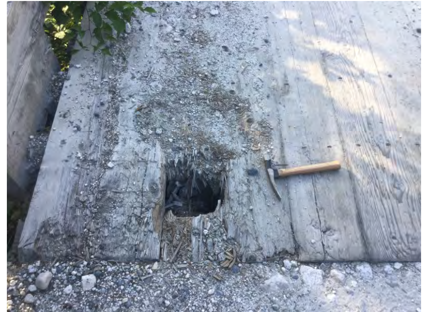
Hole in Deck at Right Abutment
