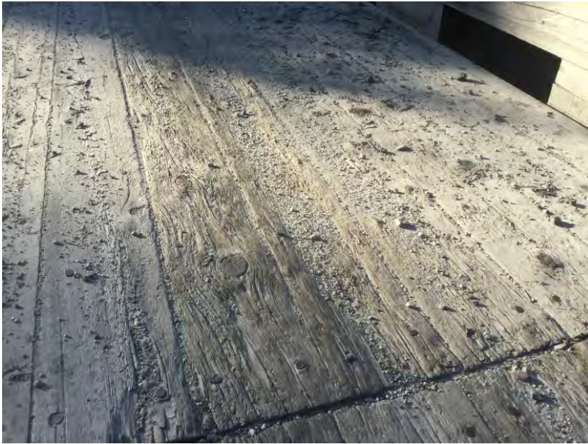
Wear in Deck
